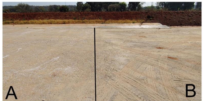
Gravel Road treated with Ge-NANO CLEARSEAL A - Treated with CLEARLSEAL B - Not treated
